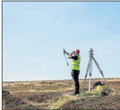
Surveying work at the site of Bilsdale transmitter, which was destroyed by fire in August
